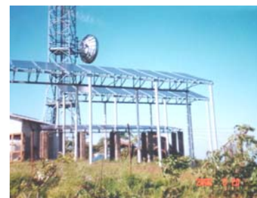
Sun-Earth brand solar modules applied in telecommunication stations.
